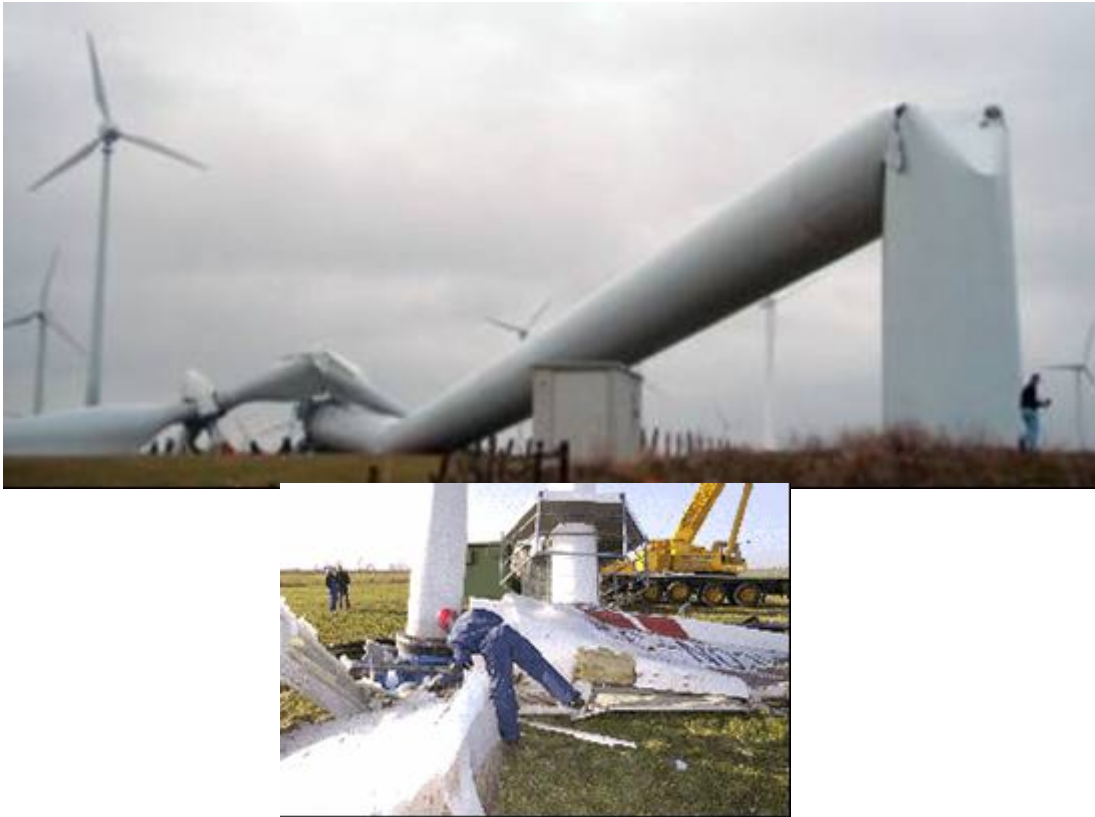
Fig. 2.1: Two examples of incidents that pose possible danger to the surrounding area.
